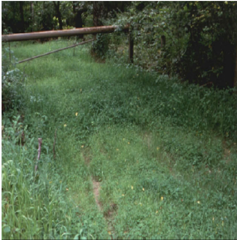
Seeding forest access roads after completion of use provides multiple benefits, including stabilizing the road and protecting it from erosion, and providing food and cover for wildlife. Seeding also eliminates negative visual impacts. Photo courtesy of Minnesota DNR
